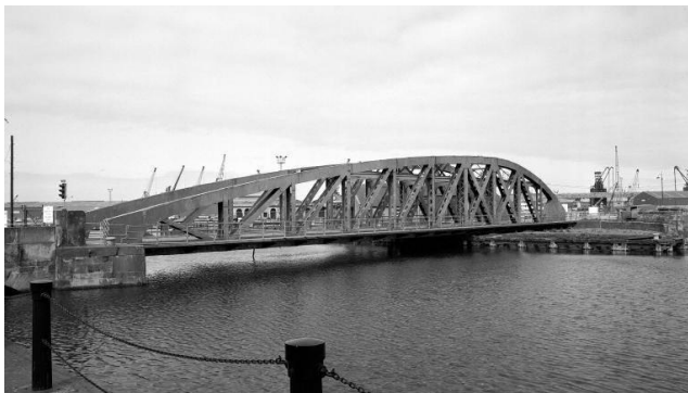
Figure 35 - Victoria Swing Bridge (F on Map 17). Completed in 1874, the Victoria Swing Bridge formed a link across the inner harbour between the Victoria Dock and the Albert Dock. At the time it was the largest swing bridge in the United Kingdom. The iron bowd-truss swing bridge in this photo is a late 19 th century replacement for the original bridge (SCRAN, 2009) (photo: c. 1970s © RCAHMS, Licensor www.scran.ac.uk).
