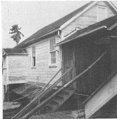
FIG. 2. LONG, BADLY GRADED ROOF-GUTTER
