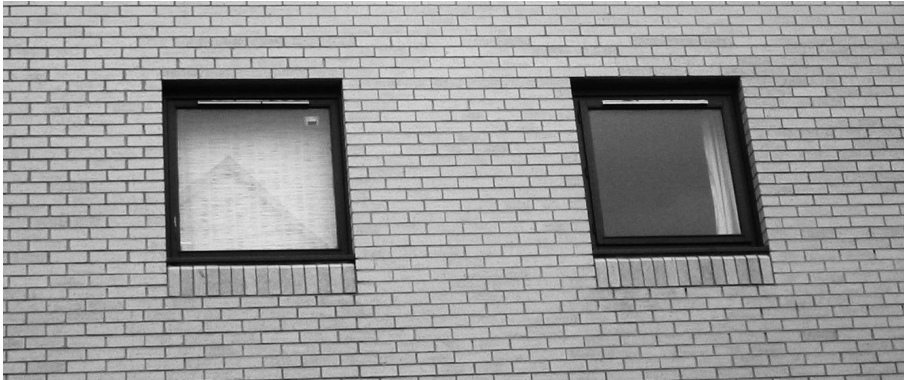
Figure 3.1: A façade of a modern brick building. The bricks form naturally rectangular openings.
