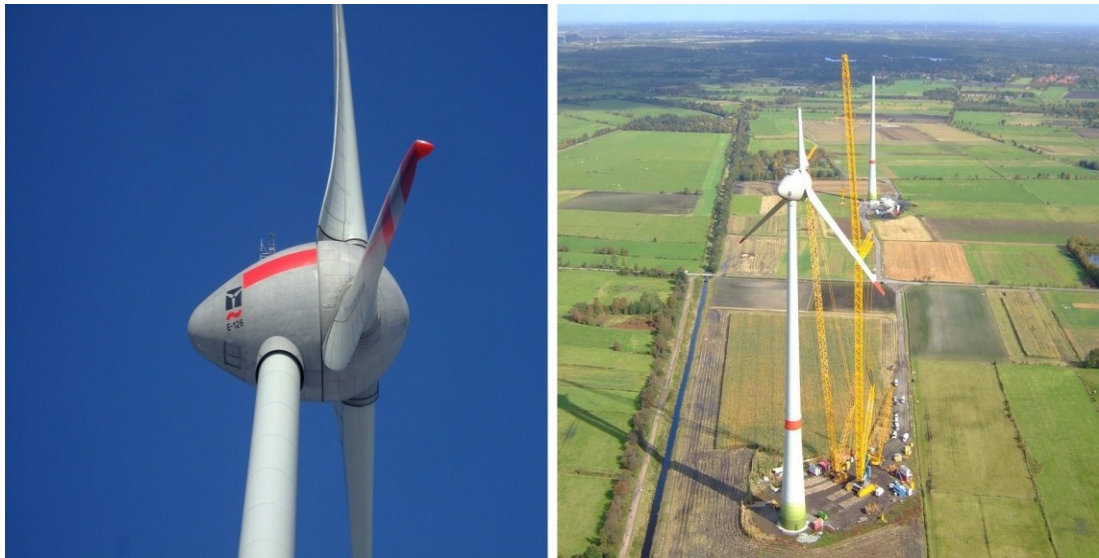
Figure 3.3 - Enercon E-126 7MW WEC [84]
