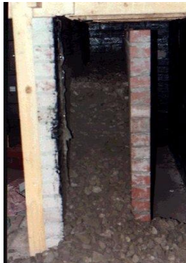
Figure 3.6 Tank containing 0.75m of spent ballast (Clark, 2001)
