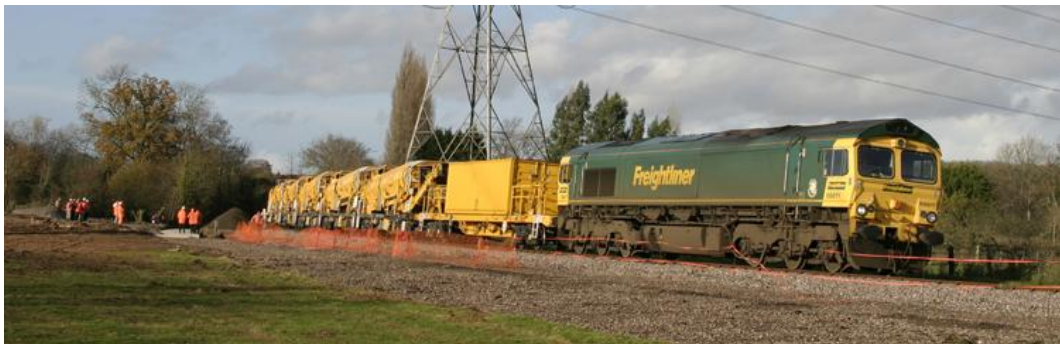
Figure 1.13 High Output Ballast Cleaner(Network Rail, 2008)
