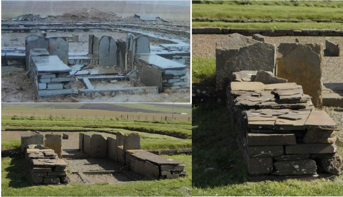
Figure 5.12a-c: Barnhouse Settlement, As initially reconstructed in 1994, and its condition today with detail of deteriorated stonework. Top left image Courtesy of RCAHMS photographic archive, 1994
