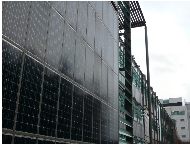
Figure 3.13: Solar photovoltaics installed at the King's Buildings, University of Edinburgh
