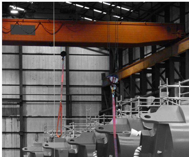
Figure 4.7: Overhead crane for PCM assembly (Photo by Ronald Parker)
