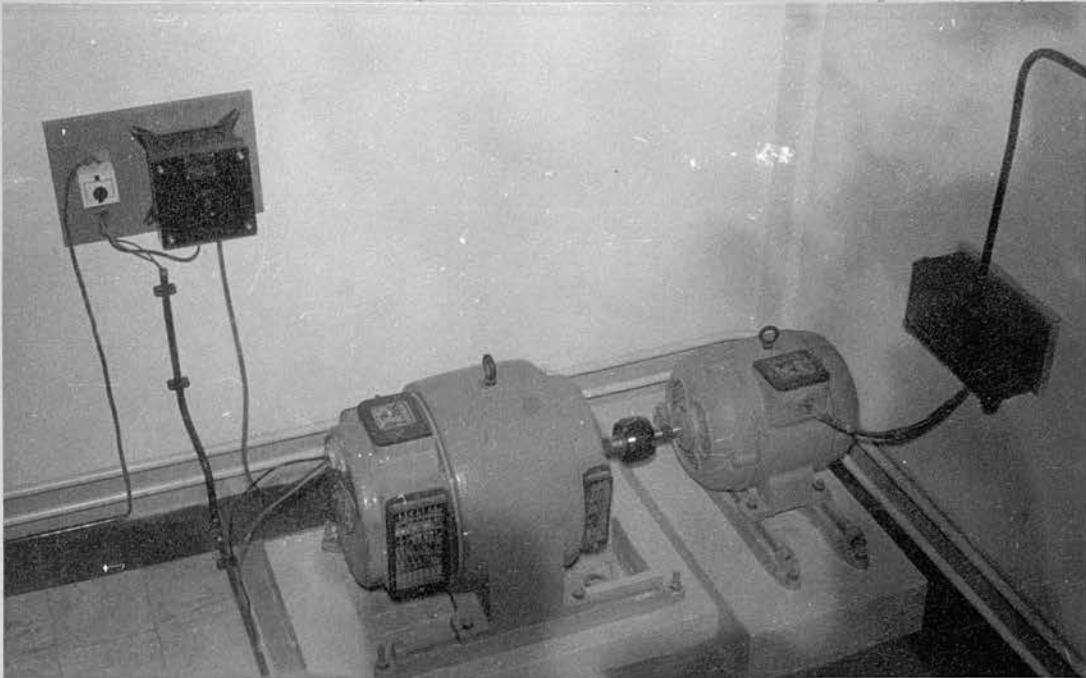
MOTOR - GENERATOR SET.
