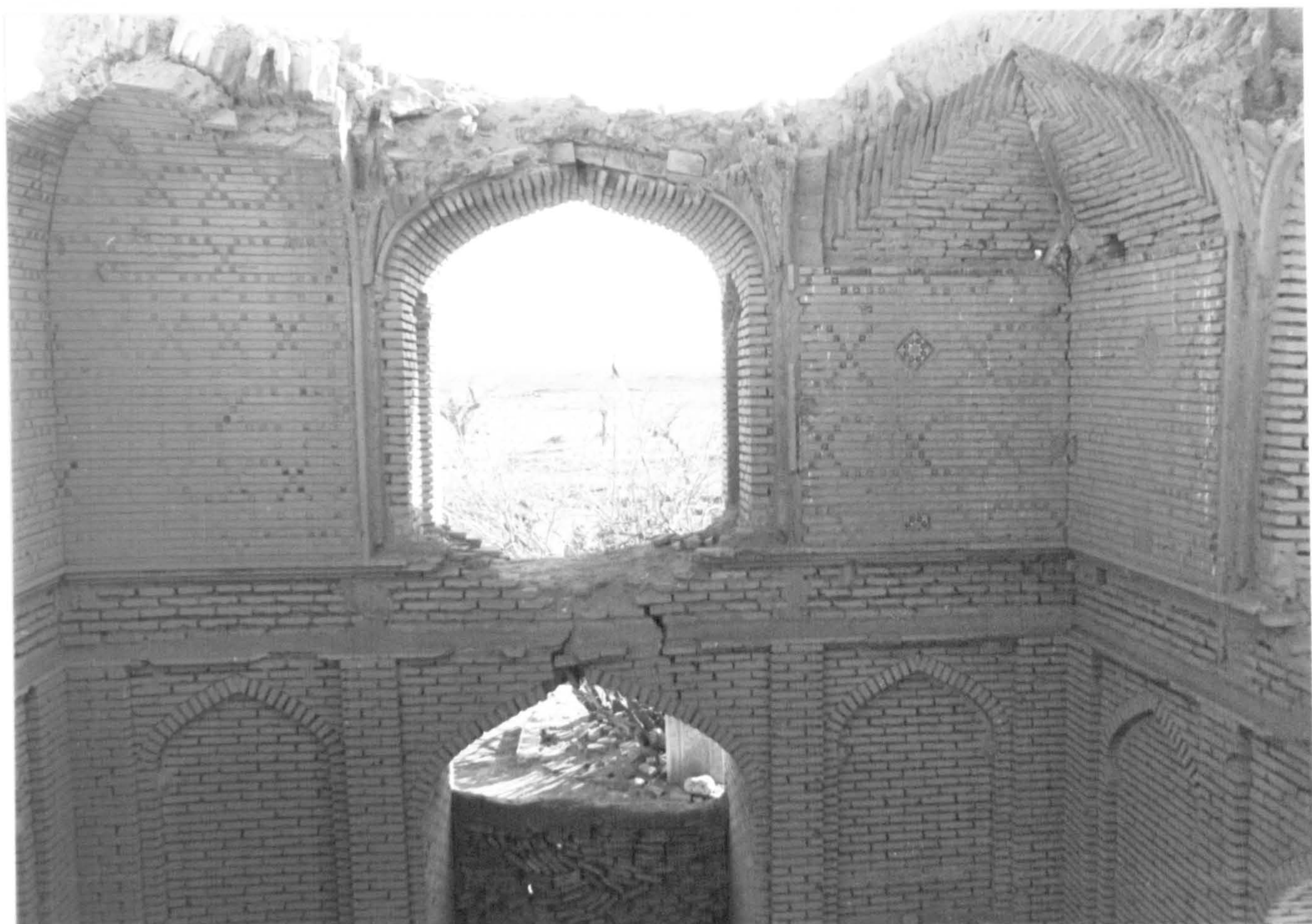
166) Dih-i Manār, Khanqah of Shaikh Armānī, interior, central dome chamber, general view
