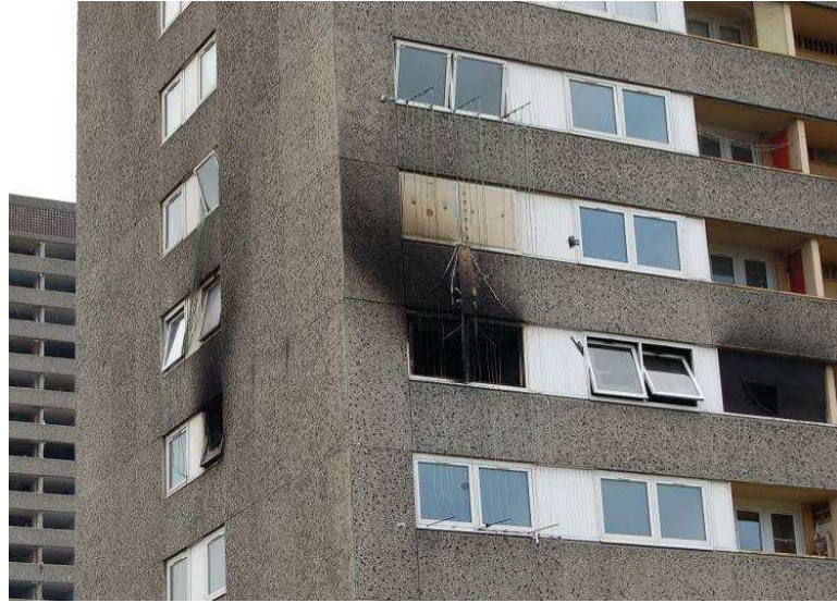
Figure 4.21. Photograph of the external façade outside Test One in the aftermath of the fire. A plume smoke record on the façade highlights the general affect of the wind on the plume tilt and shows evidence of a significant plume having emerged from the kitchen window.
