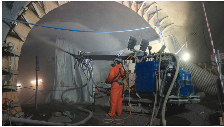
Figure 2.2: Concrete application in a freshly excavated tunnel using a 5-DoF concrete spraying unit. Image provided by Costain Laing O'Rourke Joint Venture.
