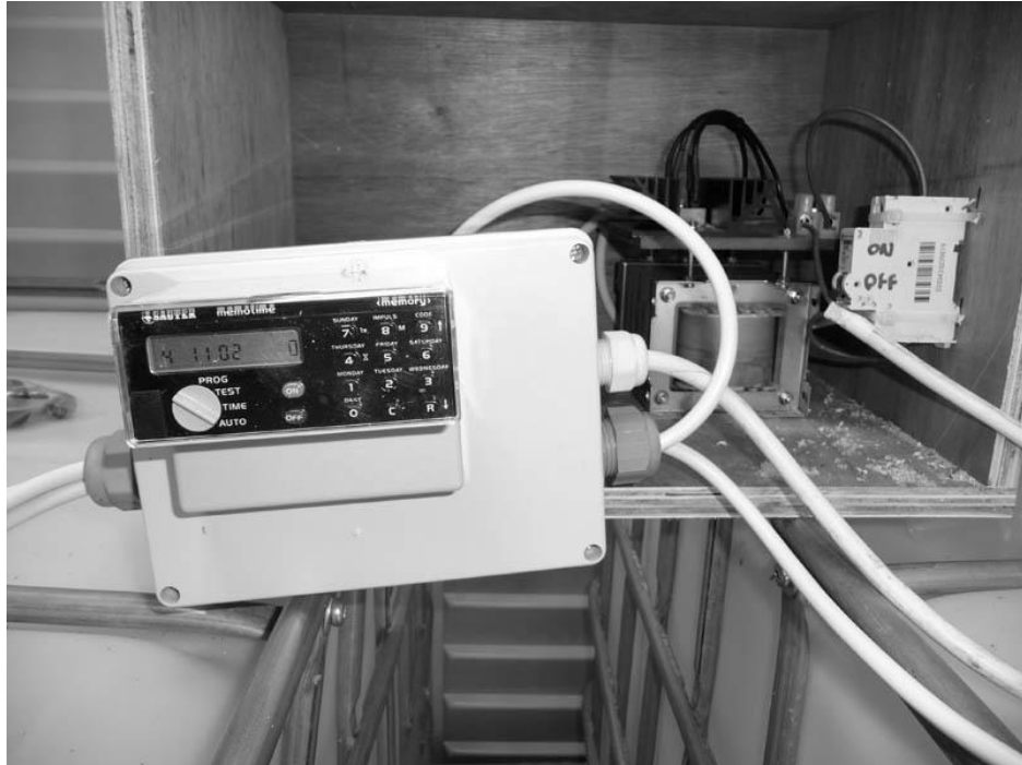
Fig 14. Updated timers fitted to pumping mechanism with master switch
