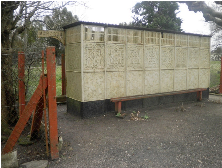
Figure 3–110. Macfarlane cast-iron urinals. Coronel Vidal Station (FCS). Source: Photo Pablo Marzilio
