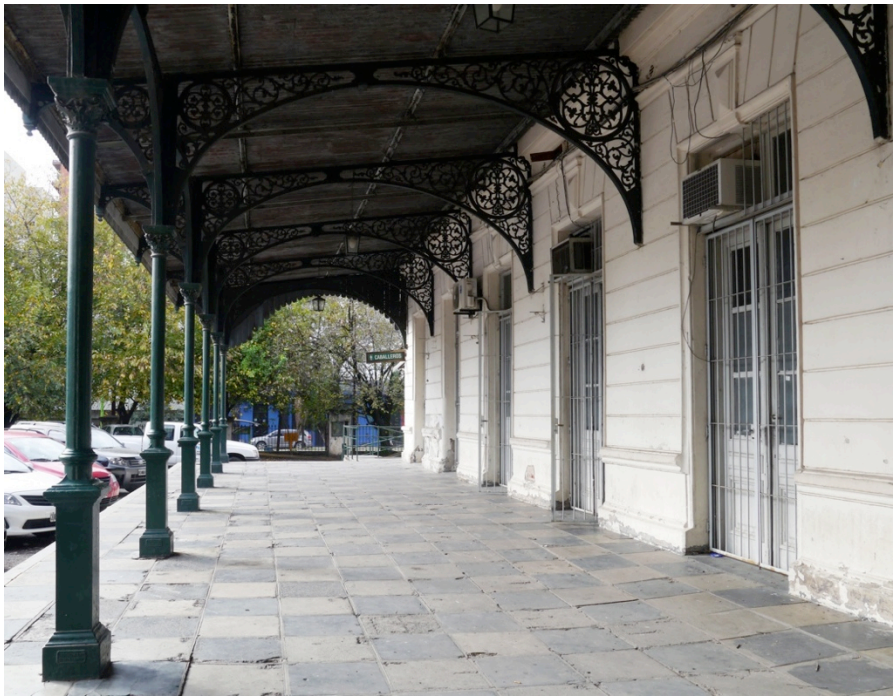
Figure 3–52. Mitre Station. Handside cast-iron brackets and columns. Source: Photo Lucia Juarez
