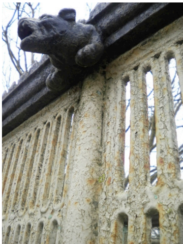
Figure 3–112. Macfarlane cast-iron urinal, detail. Coronel Vidal Station (FCS). Source: Photo Pablo Marzilio
