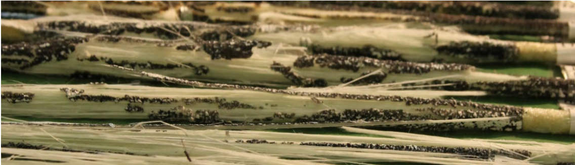
Figure 4-25 Splitting of sand coating on bar PTG at T_g, Modulus , due to transverse thermal expansion of the FRP
