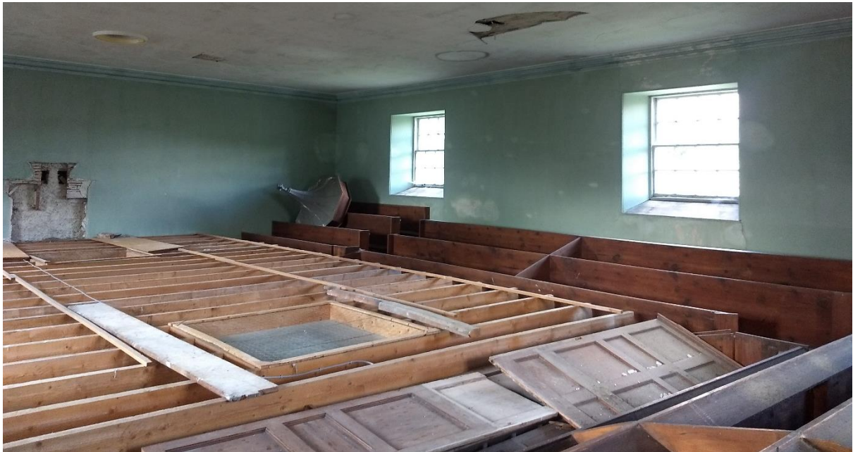
Figure 38. View of the upper gallery, closed off by a false ceiling since the 1950s (Photo by author)
