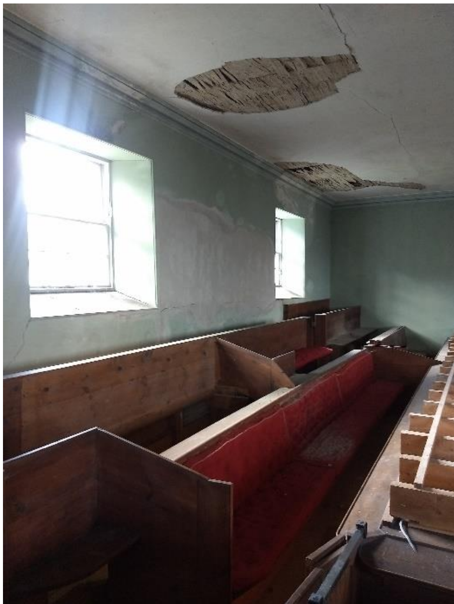
Figure 40. View of upper level interior, highlighting fallen plaster from the ceiling and cracking and staining on the wall (Photo by author)
