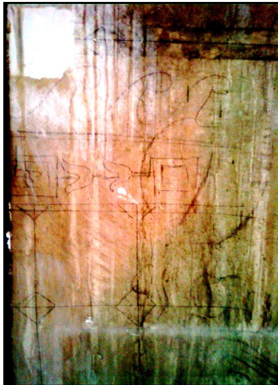
Figure 1.2. The building as archive: pencil sketches for decorative scheme on the wall behind display case removed from east wall of the first floor of the West Wing during Royal Museum Project. The sketch was subsequently obliterated (photograph by the author, 9 August 2010).
