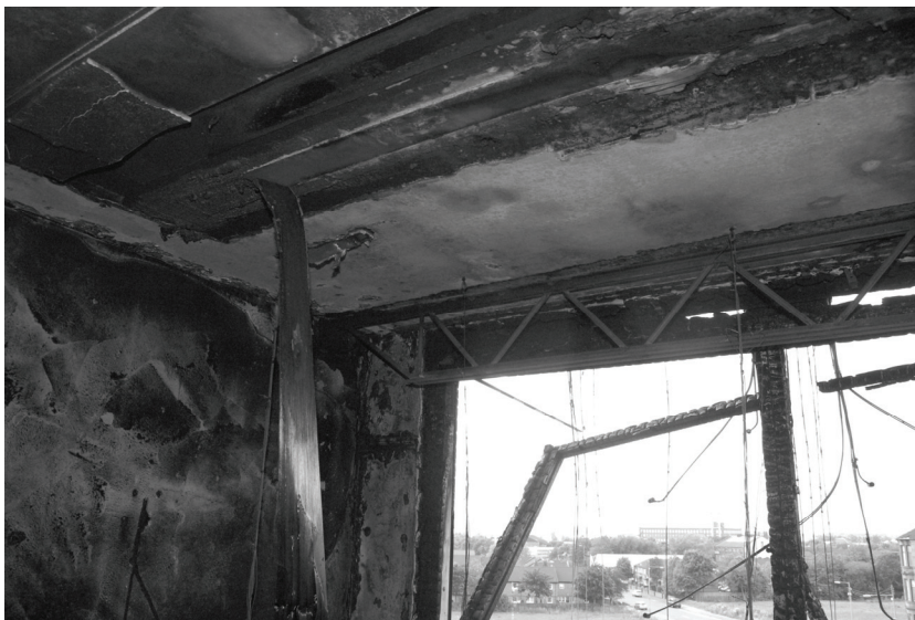
Figure 5b: Remains of intumescent-protected plate
