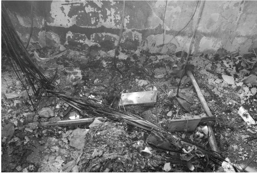
Figure 5a: Remains of unprotected plate
