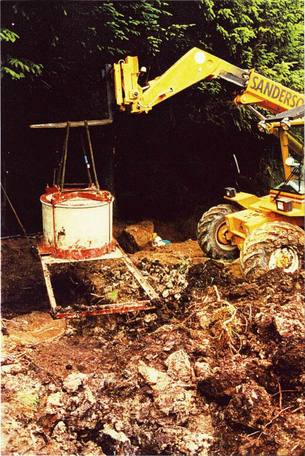
Plate A1.3. Removing the monolith from the pit. The monolith with steel under-cutting frame attached is hoisted out of the pit by a front-loader.
