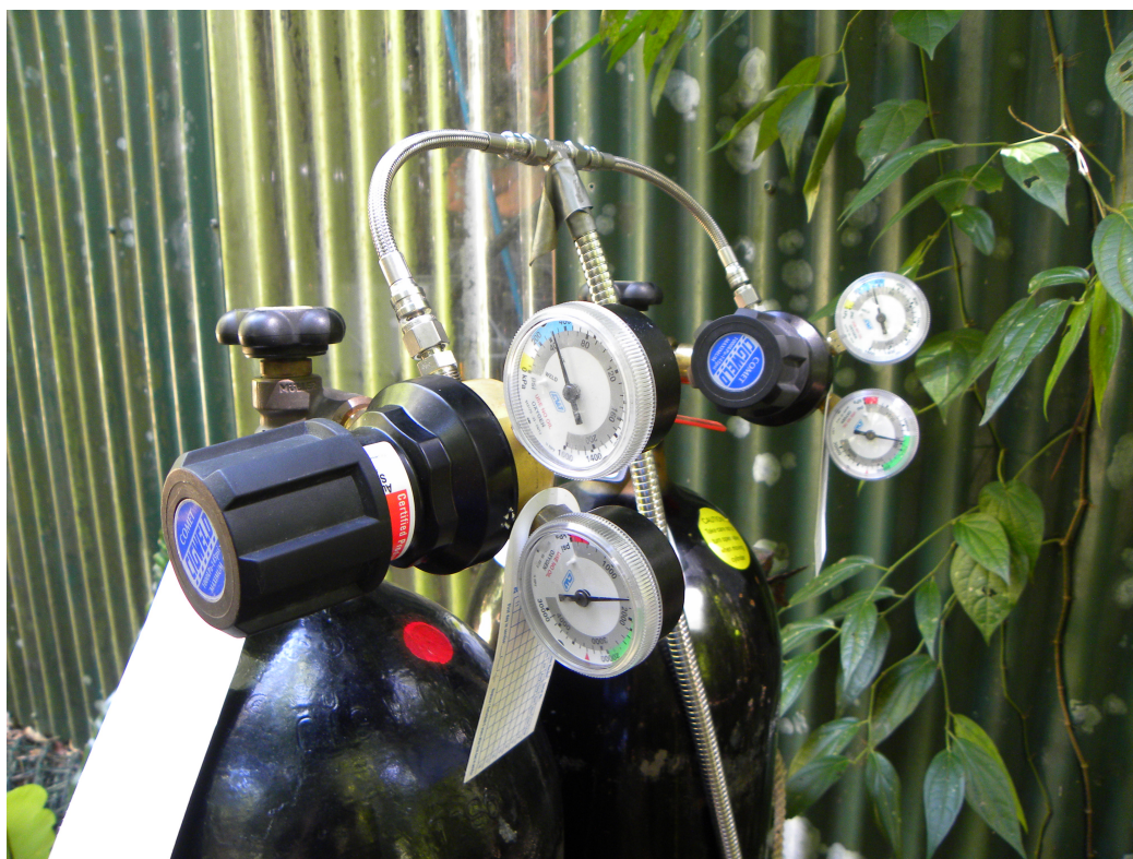
Figure 2.10: The two oxygen tanks are joined in a T, which then continues inside to the FIS. The arm sections of the lines are Swagelok stainless steel, and the main body of the line is 1/4" teflon encased inside a flexible steel plumbing line. All joints are tested for leaks every 5 weeks when tanks are replaced. The entire assembly is then covered in plastic to protect from rain.
