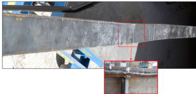
b) Top view of the of the control beam after testing with the distorted top flange
