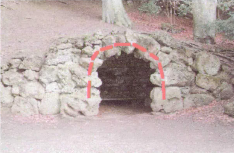
Figure 3.2: Example of a key-stone structure, an arching effect. The downward force of the over-burden spreads out to the stones on either side of the keystone. The red lines indicate the direction of the inter-block normal forces.
