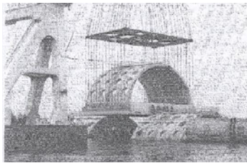
(e) Semicircular caissons was towed to the construction site by a floating crane
