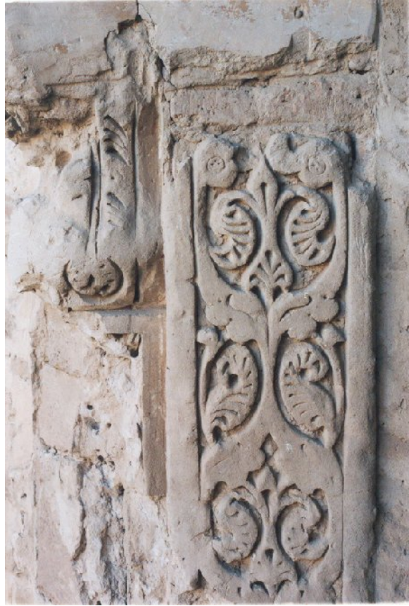
Pl.6.7.Friday mosque at Ardistan. Remains of carved stucco in upper storey.
