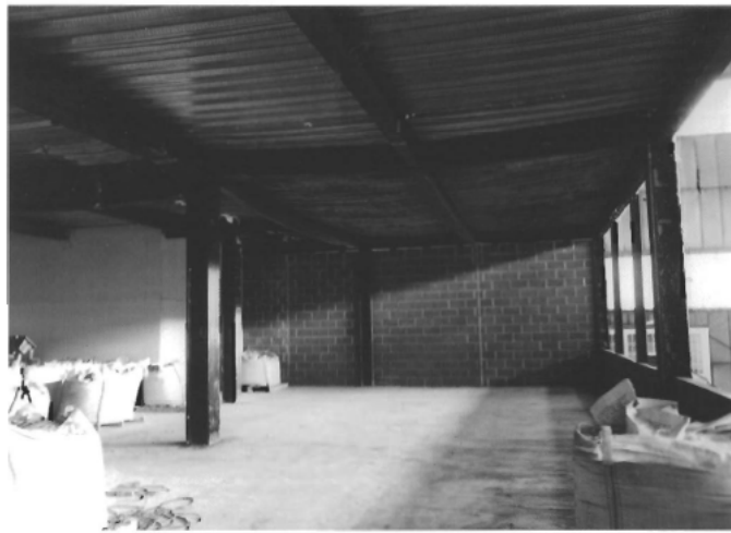
Figure 2.16: Internal view of Post-test deformation of BS corner test (BS, 1999)
