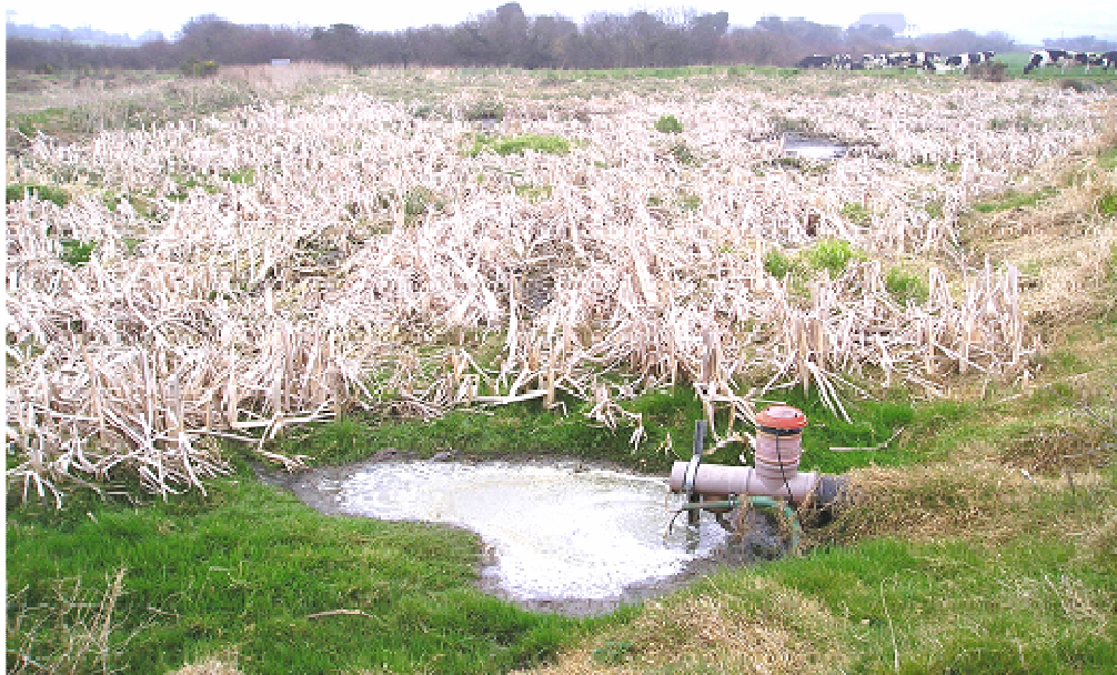
Figure 4-4. Main inlet of integrated constructed wetland 11 (cell 1), Waterford, Ireland (February, 2007).
