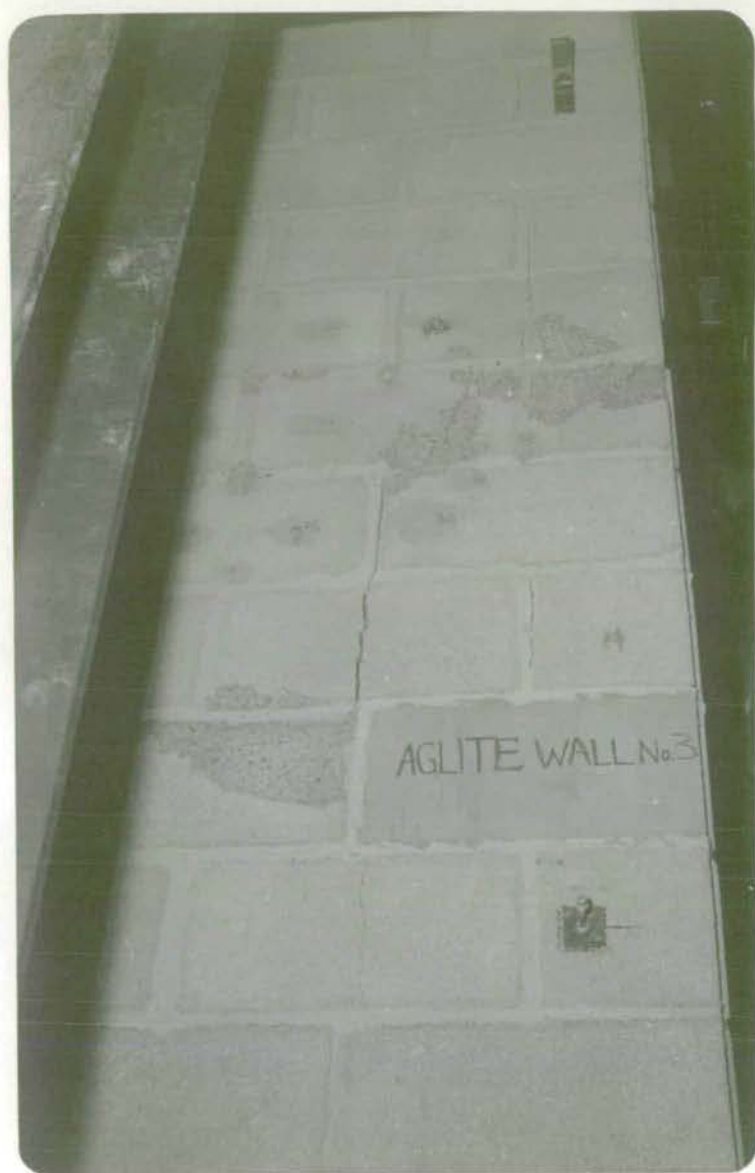
Plate 3.13 TENSILE SPLITTING FAILURE IN FULL SCALE "AGLITE" BLOCKWORK
