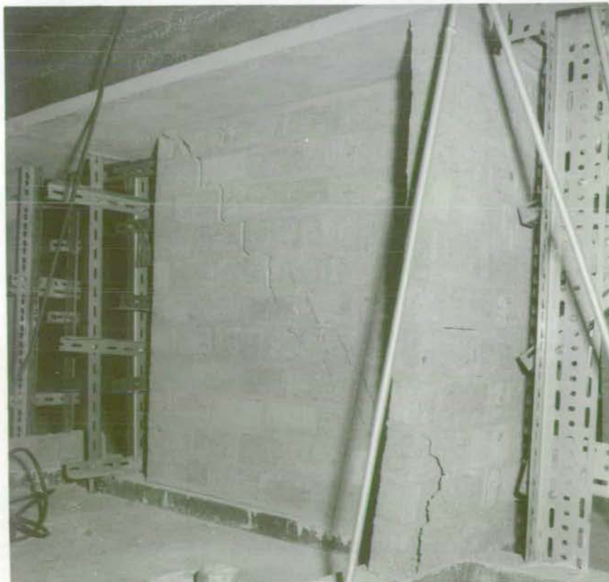
Plate 4.11 FAILURE OF SINGLE STOREY BLOCKWORK SHEAR WALL UNDER LATERAL LOADING AT 100 \text{ lbf/in}^2 PRECOMPRESSION
