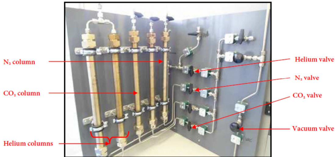
Figure 5.7 Drying columns and control valves
