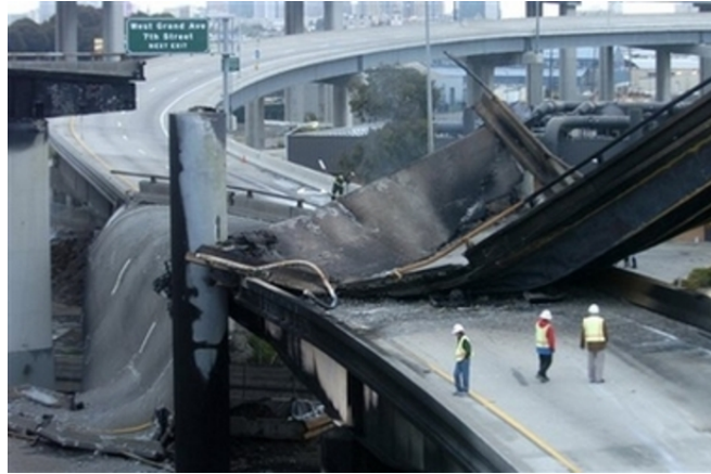
Figure 2.14: A bridge partially collapse after a fire
