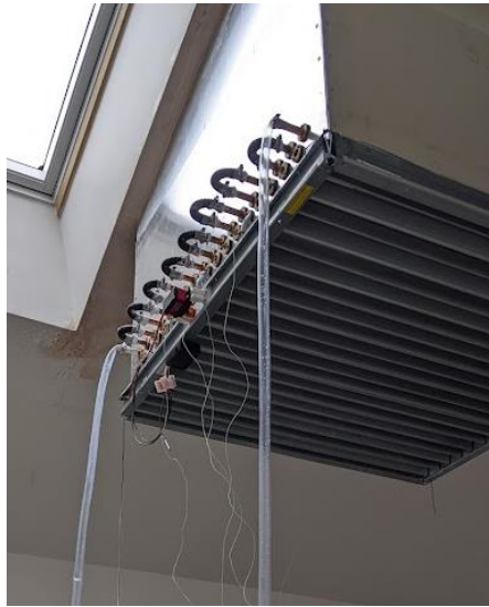
Figure 5-3 - Copper pipes installed through the wind tower ducting inside the test room
