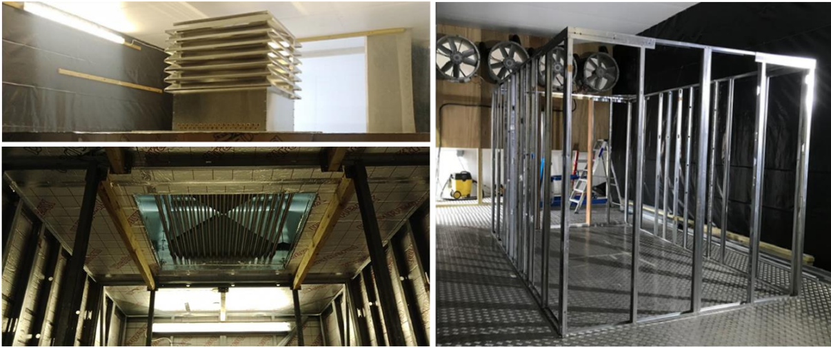
Figure 4-6 - Wind tunnel experimental set up showing wind tower on top of test room (top left), heat pipes through base of wind tower (bottom left), and test room frame inside the constructed wind tunnel test section (right)
