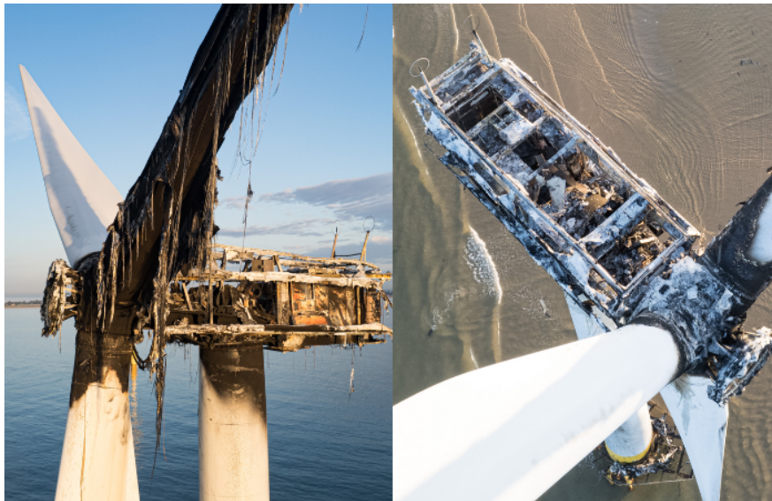
Figure 2.2: Wind turbine after the fire on one of the Scroby Sands (UK) wind farms. Source: Oliv3r Drone Photography (4C Offshore, 2023c)
