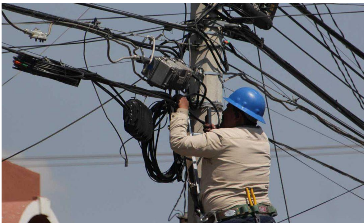
Figure 2 - CFE worker maintaining old and inefficient electricity infrastructure in Mexico. (El Universal, R, 2023)
