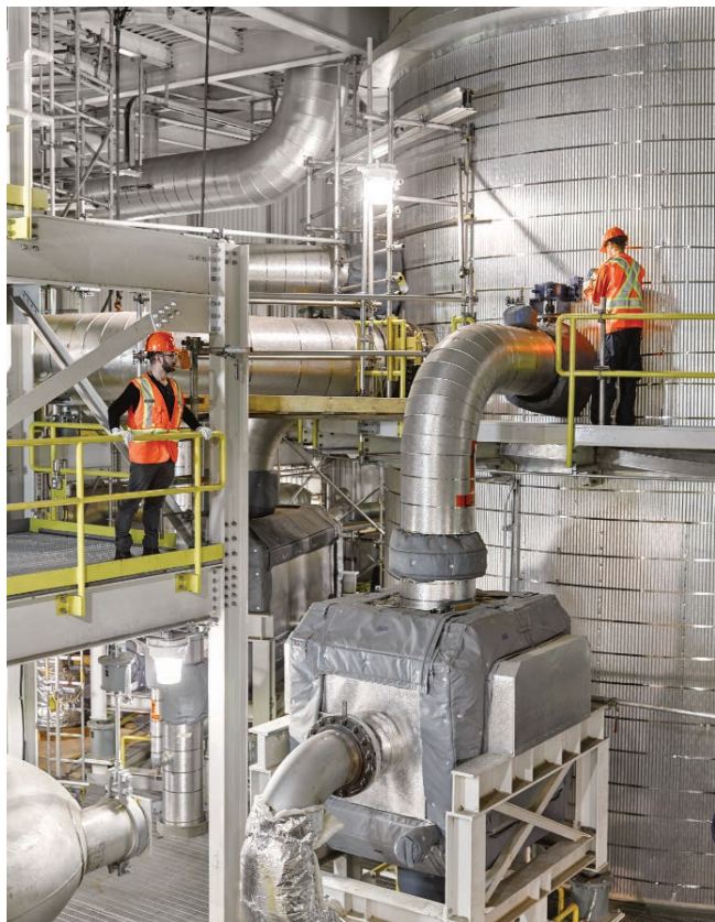
Inside the Boundary Dam CCS facility. Photo courtesy of SaskPower
