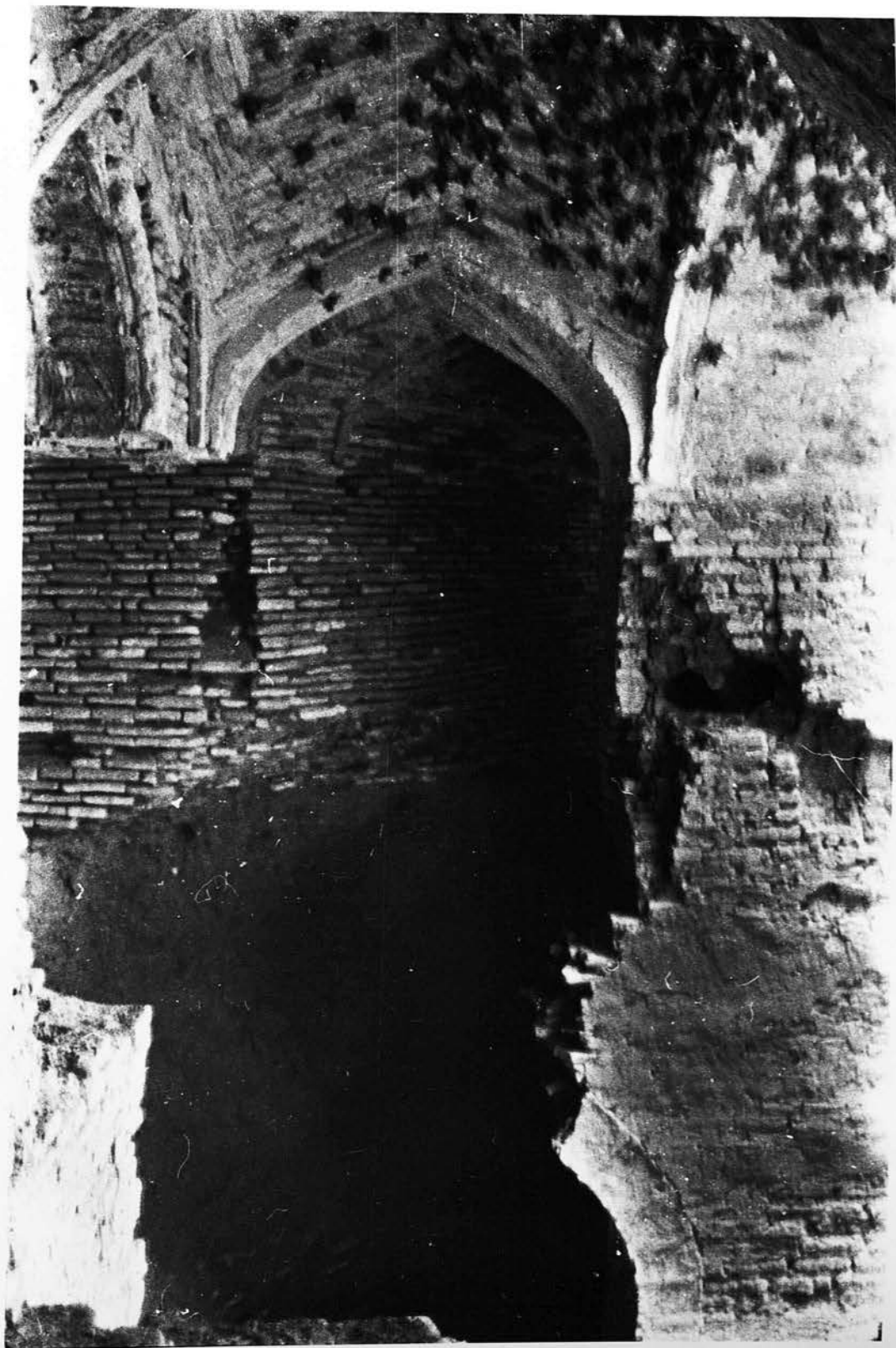
160-Bost Afghanistan;The Well, Levels 2 and 3 ; Coridors 39 and 53 (the roof of ThoLevel 3 is collapsed ) .
