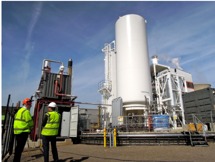
Figure 2.25 Highview's 350kW liquid air energy storage demonstration project (source [85])
