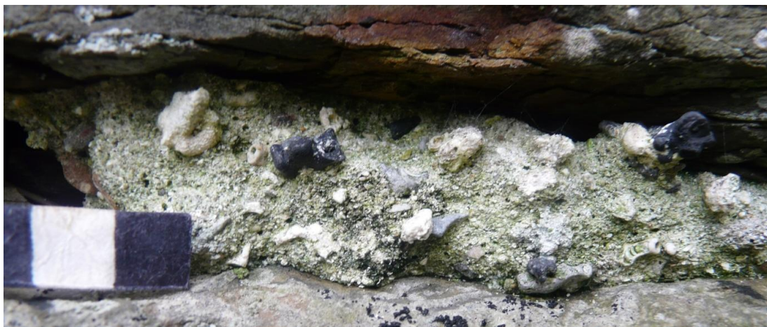
Figure 3.18 (above) – Range of altered maerl clasts in primary bedding mortar at St Mary's, Wyre, Orkney. Scale 10mm; photograph M. Thacker.
