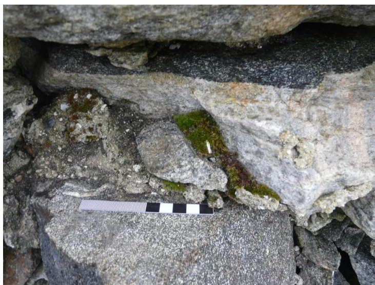
Figure 5.4 (above) – Important fragments of core mortar survive in-situ, binding rubble to the back of a face stone. Despite surviving as an almost completely dry-stone structure in which the beds are also largely devoid of mortar, this church was evidently formerly fully lime-bonded. Teampull Choluim Chille , Benbecula. mm and cm scale; photograph M. Thacker.
