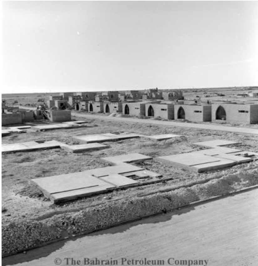
Image 5.10. Isa Town Houses in their various stages, with the foundations ready for inspection. Source: BAPCO Energies.
