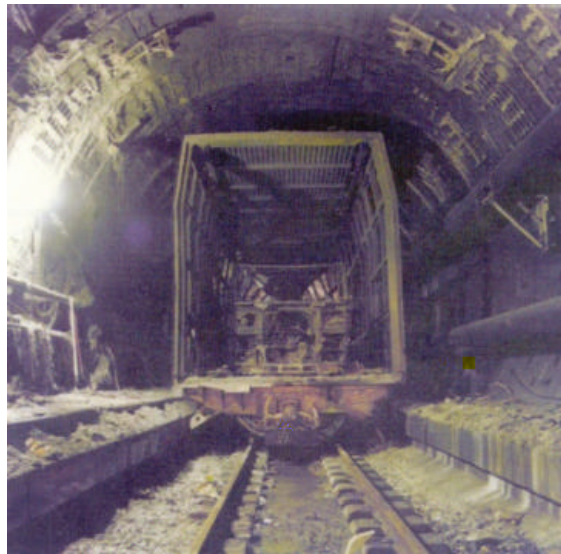
Figure 1.01 – The aftermath of the Channel Tunnel fire (18.11.96) [20]
