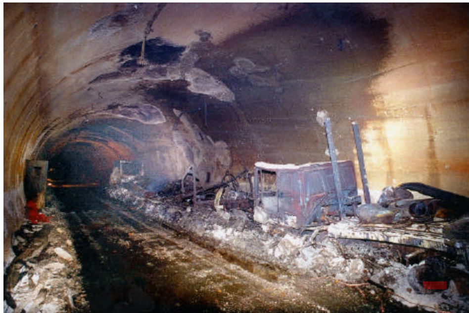
Figure 1.03 – The remains of the vehicles after the Mont Blanc tunnel fire (24.3.99)
