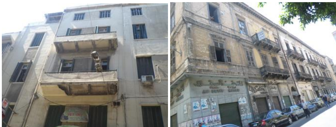
Figure 53. building in relatively bad condition.
