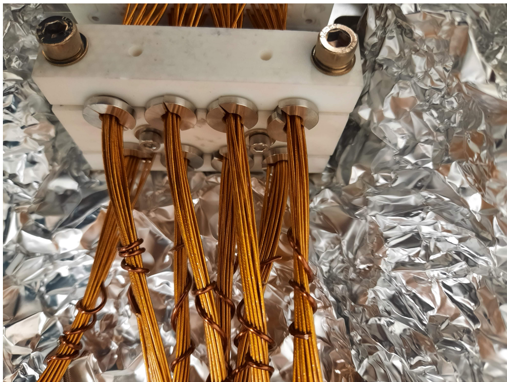
Figure 3.6: Close up view of the MACOR strain reliefs mounted to the cable harnesses. Kapton cables are separated into bundles of 8-10 wires to be fed through strain relief. Additional stainless steel funnels were placed within strain reliefs to reduce cable stress.
