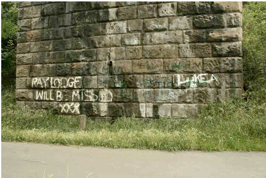
Figure 13.6 Graffiti on Five Arches Bridge (July 2009).
