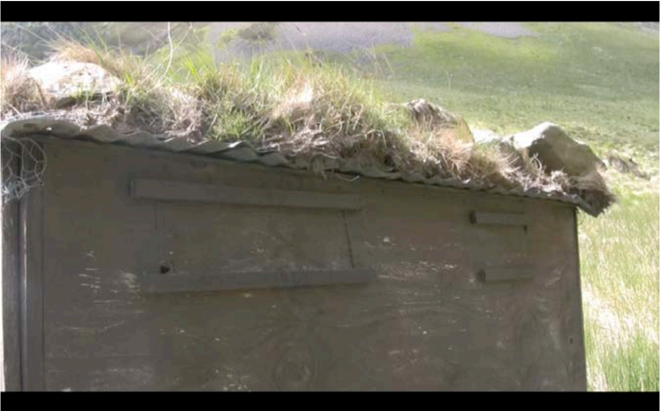
Figure 11.22 Deer stalker hut. The corrugated iron roof is visible under the turf (June, 2010).
