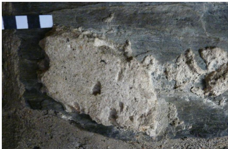
Figure 5 (above) - Probable Mortar 3 remains on face of south wall of Columba's shrine. This structure clearly requires more work. Scale 10mm; photograph Mark Thacker.
