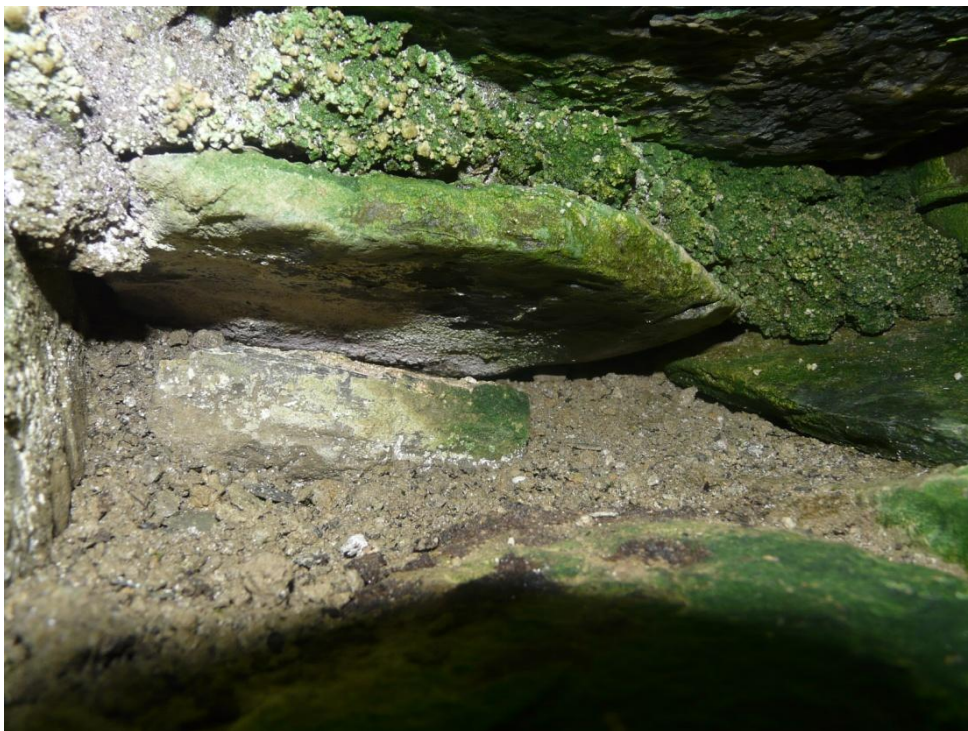
Figure 11 (above) – Crosskirk Tuquoy. Degading mortar binding core rubble; east of south nave putlog. No scale; photograph Mark Thacker.
