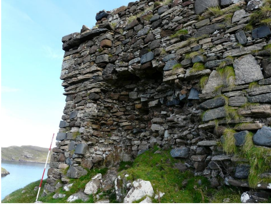
Figure 8 (above) – Collapsed face of south-west enclosure wall near west corner. The ranging rod is at the same angle as battered wall profile. Scale 500mm; photograph Mark Thacker.
