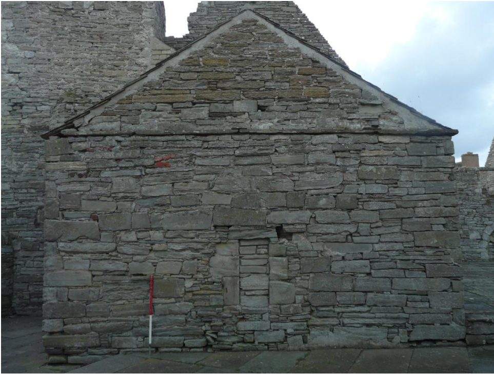
Figure 3 (above) – Chancel; East wall; external face. Note disturbed masonry around the secondary window and large void where Mortars 1 and 2 are visible in core contexts. Scale 500mm; photograph Mark Thacker.
