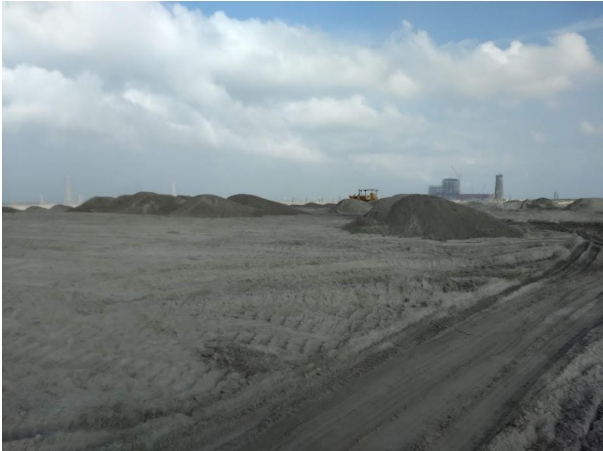
Figure 13. The ash road that led up to the under construction TANGEDCO power plant in the distance. It was a dicey ride, worsened by pools of water that stagnated in lower ground with the late October rains.
