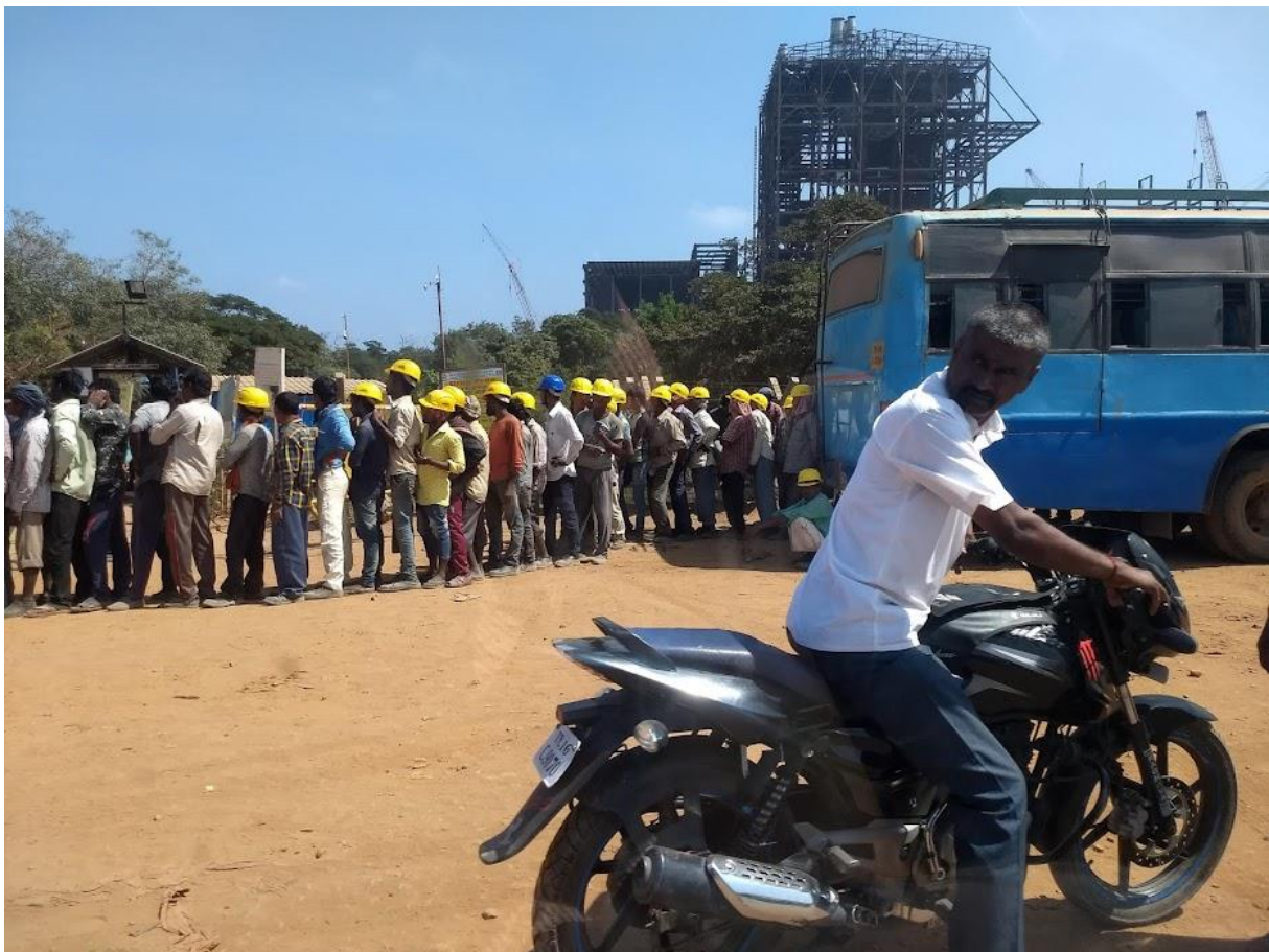
Figure 12. A long queue of workers standing by the construction site of the NCTPS phase 3, waiting for their identity cards to be checked by the private security personnel manned at every entry/exit gate.
