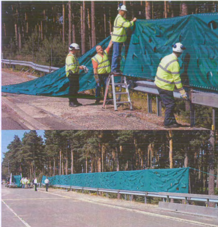
Figure 5.10 Photographs of a new portable incident screen system (Source: Mr. Bob Wadsworth).
