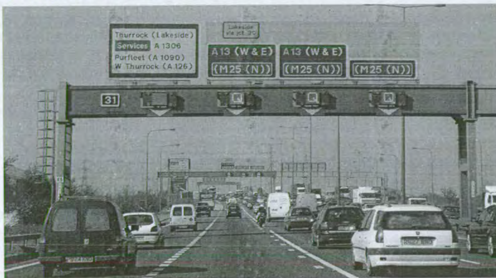
Figure 2 Example of gantry matrix signals.
