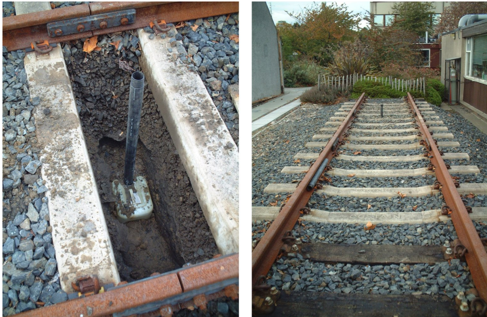
Figure C-2. Photo of the canister (left) and of the trackbed after the insertion (right)
