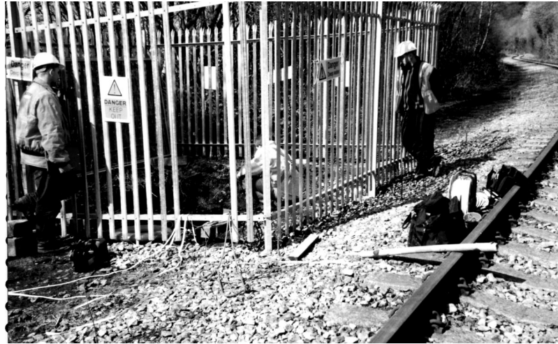
Figure 2.7. A mineshaft collapse in proximity of the railway near Machen, in South Wales in 2001
