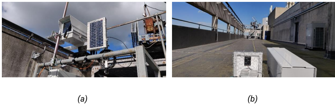
Figure 6-30: Installation at the JCMB, King's Building, University of Edinburgh
