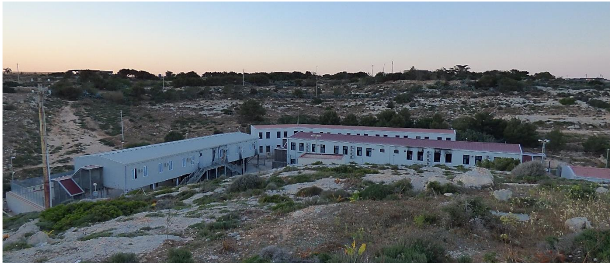
Figure 8 - Lampedusa's reception centre in April 2018; fire damage is evident just right of centre on the façade of the left-hand and the front-right blocks.
