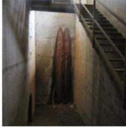
Figures 4.16 and 4.17 A tunnel was built under the dam wall of Pawe Diga to facilitate river-crossing. Today the tunnel is dark (defunct generator) and several leakages have filled it with water. Brave people still use it nonetheless.
