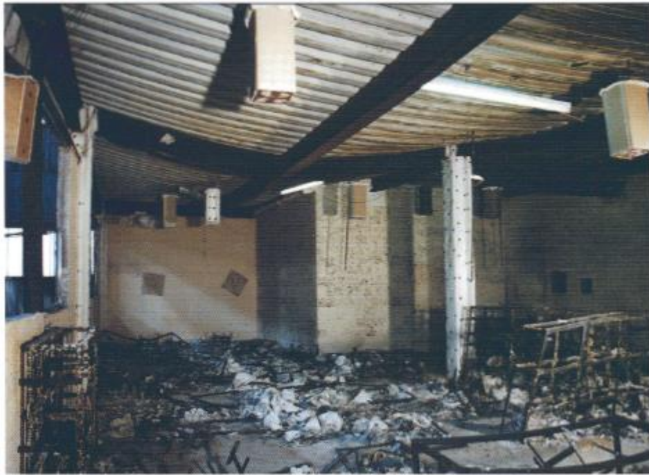
Figure 2.9. Internal view of British Steel test 6 showing large deflections of the floor above (British Steel, 1999)
