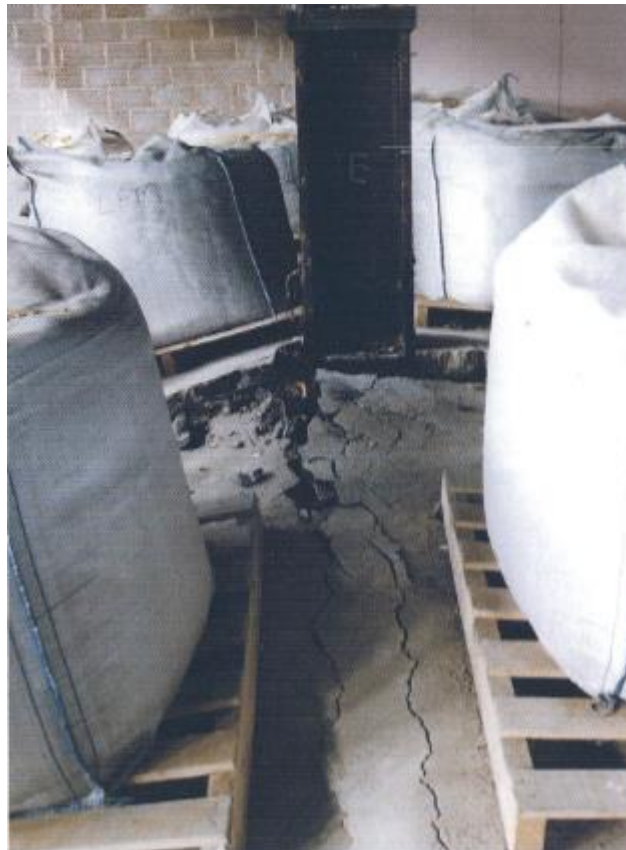
Figure 2.10. Internal view showing cracking of the composite slab over support line from British Steel test 6 (British Steel, 1999)
