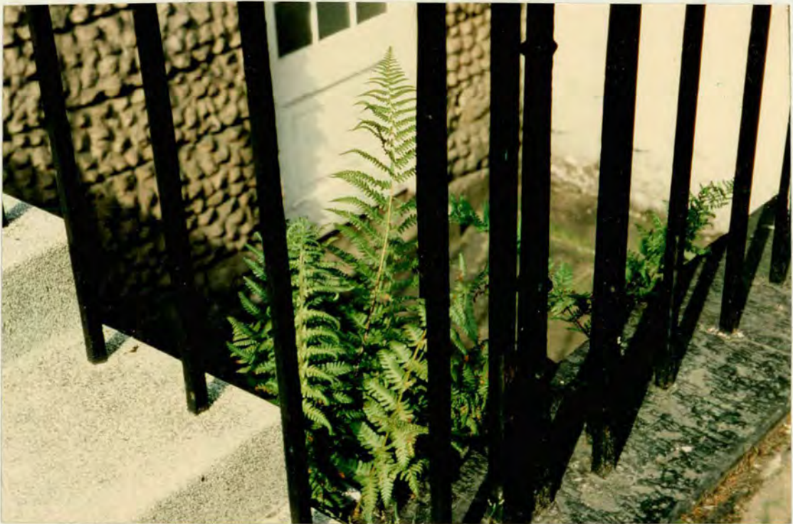
Figure 5.1 Dryopteris filix-mas growing on a basement wall in Edinburgh's New Town.
