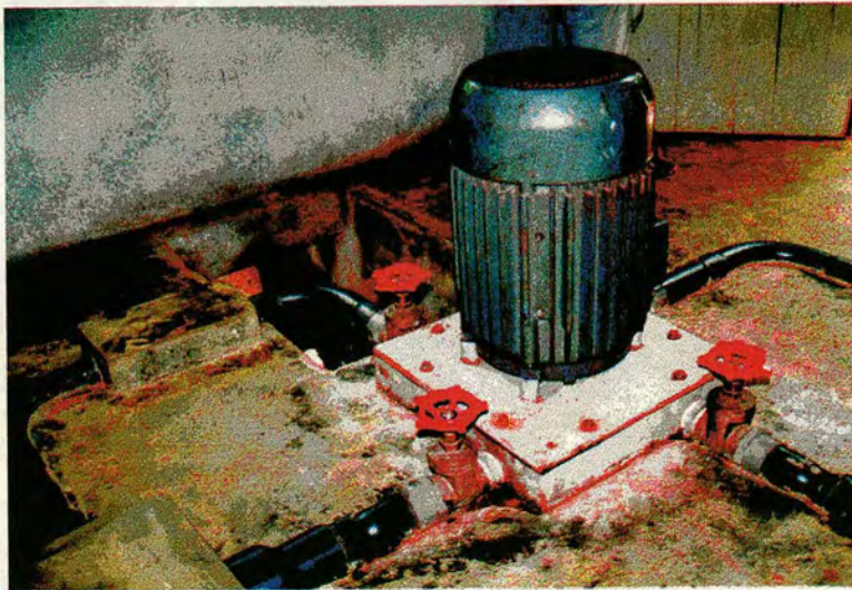
Figure 4.5: Typical IT village micro hydropower turbine and generator
